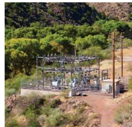
There is a substation at Childs, but the power plant is gone.
